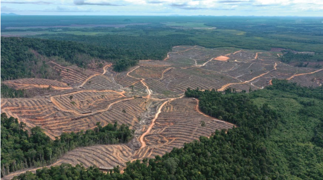
Land clearing operations in PT Mayawana Persada’s concession in preparation for industrial-scale pulpwood plantation development, July 2023.
